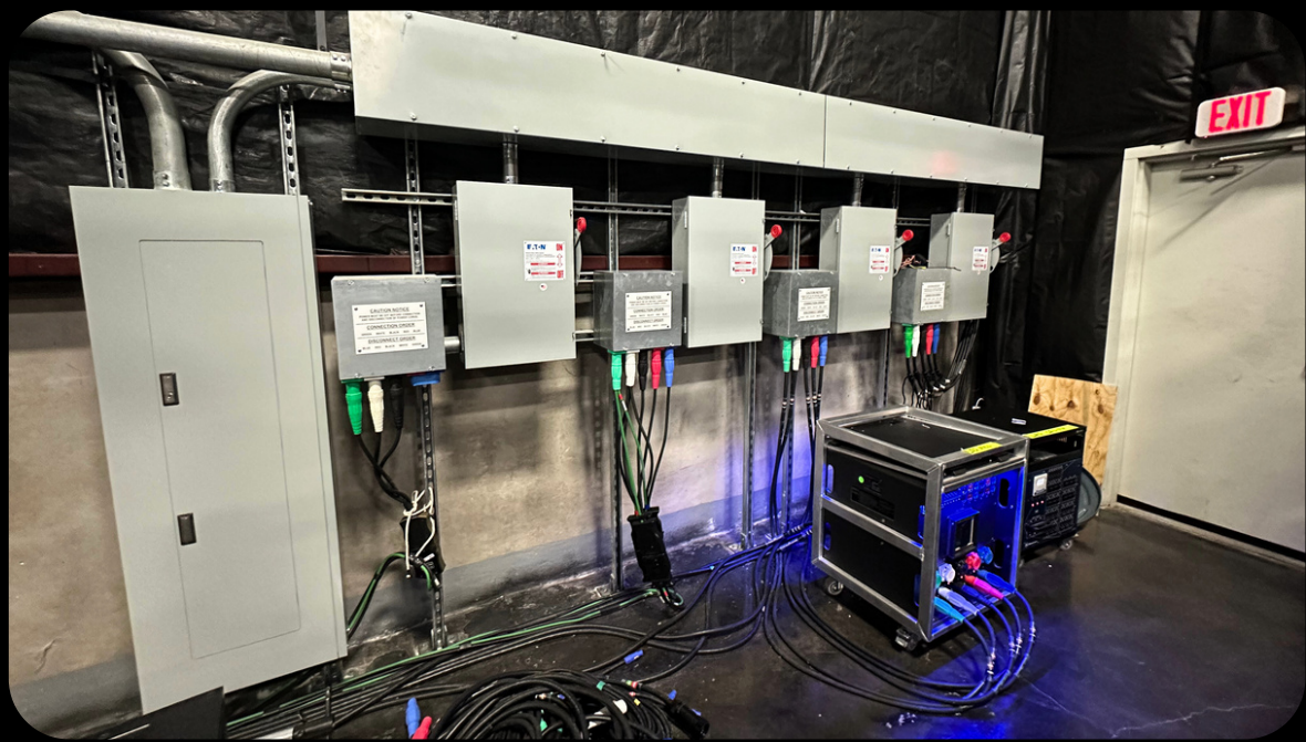
800 AMPS OF 3-PHASE SHOW POWER
